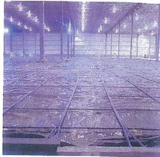
A 340x125-foot distribution center floor slab with two-way bundled PT tendons and no joints or cracks after eight years. Note void former offset so that bollard will be centered after 1 inch plus of slab movement.
