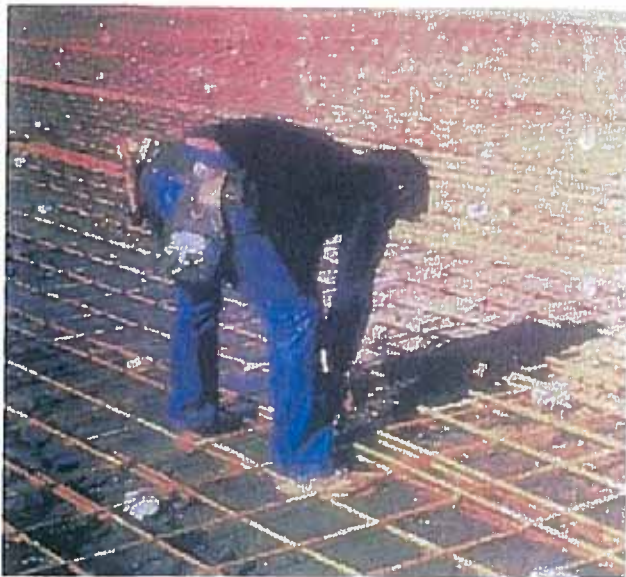
Heavy continuous reinforcing to eliminate contraction joints and only have tight cracks.
