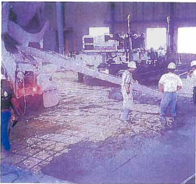
Light reinforcing continued through contraction joints for load transfer and chained up just before concrete placement.
