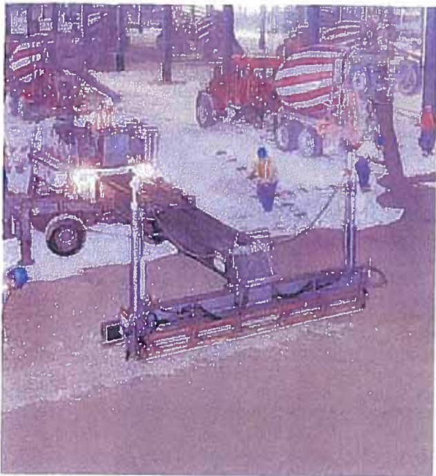
Tapered plate dowel baskets being installed just ahead of concrete placement at contraction joint location painted on base.
