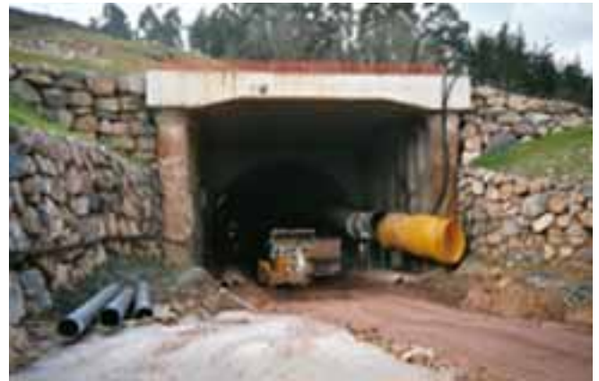
Over 30,000 lbs. of FORTA-FERRO® fiber were used to line a tunnel for the city of Navarre, Spain.
